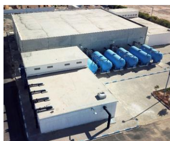
Water desalination and demineralization of brackish water and potabilization
