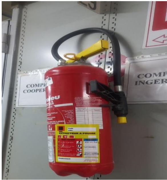
Figure 14: Fire extinguisher in the warehouse
